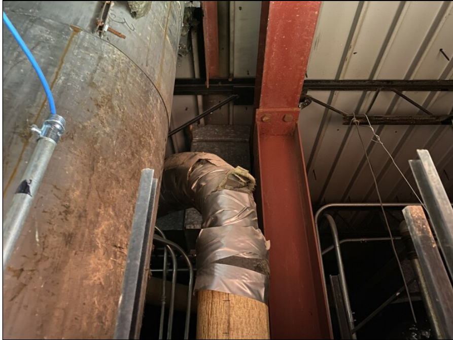
7 - View of fiberglass piping.
