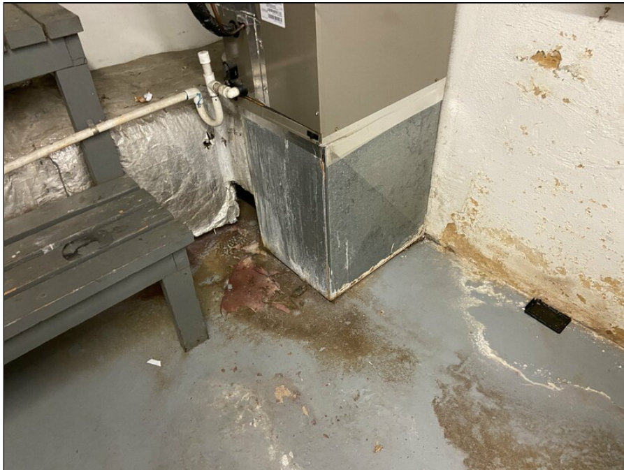
8 - View of water damage on basement floor
