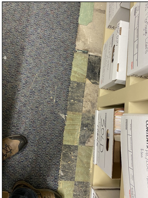
4 - View of asbestos-containing black floor tile
